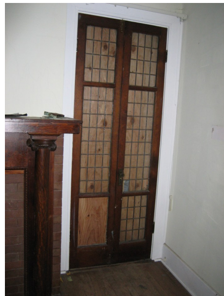
Leaded glass doors in Bemis House are missing panes and boarded up.
